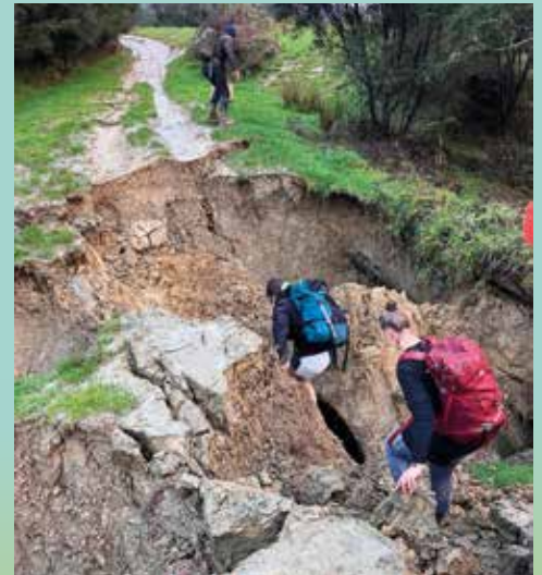
THE SPOT ON NGATOTO RD WHERE FLOODING HAS BLOWN OUT A CULVERT.
